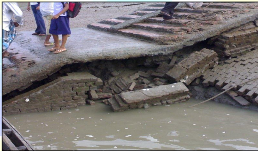
Plate 1: Erosion due to undercurrents at the ferry ghat near Basanti Bazaar, 2008
